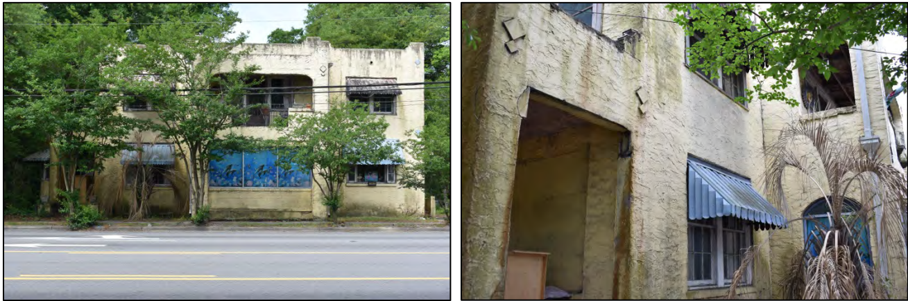
Figure 6: At left, east front elevation; at right, detail of elevation, depicting added one-story section to left and balcony to right
