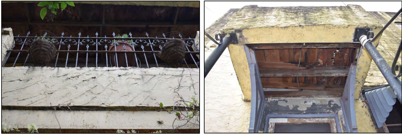
Figure 10: East front elevation balcony supported by steel beam and protected by decorative metal balustrade, at left, and bracketed hood over north side entry, at right
