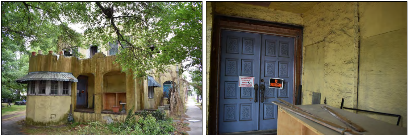
Figure 9. At left, south side and east front elevations; at right, detail of south side elevation with modern doors and boarded-over bays
