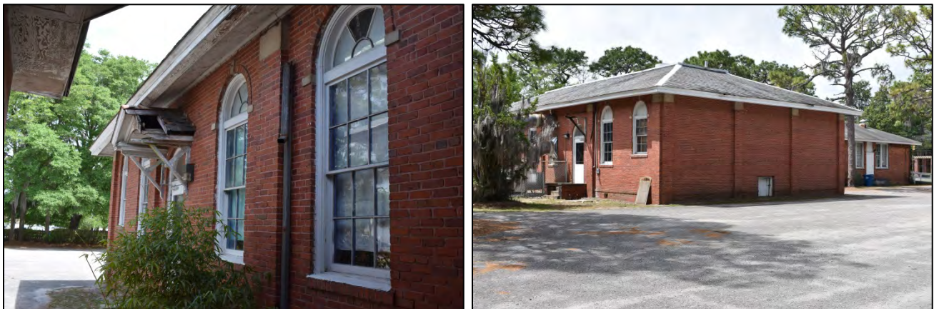
Figure 34: At left, west elevation of auditorium and, at right, east rear and north side elevations of auditorium/classroom addition
